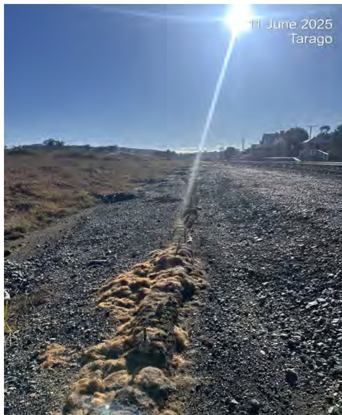
Photo 12: Damage to sediment control coir logs between southern and middle culverts.
