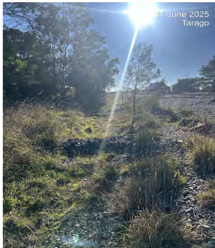
Photo 11: Rock armoury in drainage channel between southern and middle culverts. Minor sediment and vegetation buildup within drainage line.
