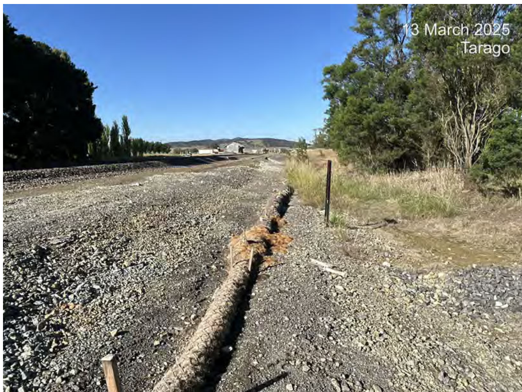
Photo 12: Damage to sediment control coir logs between southern and middle culverts.
