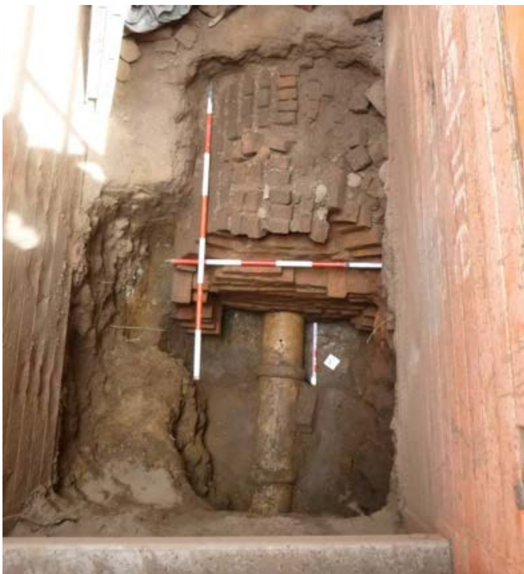
Figure 36 - Vertical view of the blocked drain in Sondage 6. South is to top of image. Note the 'slumping' of the bricks at the crown of the drain indicating the collapse which blocked the drain and required physical intervention. (Source: AAJV 2018)
