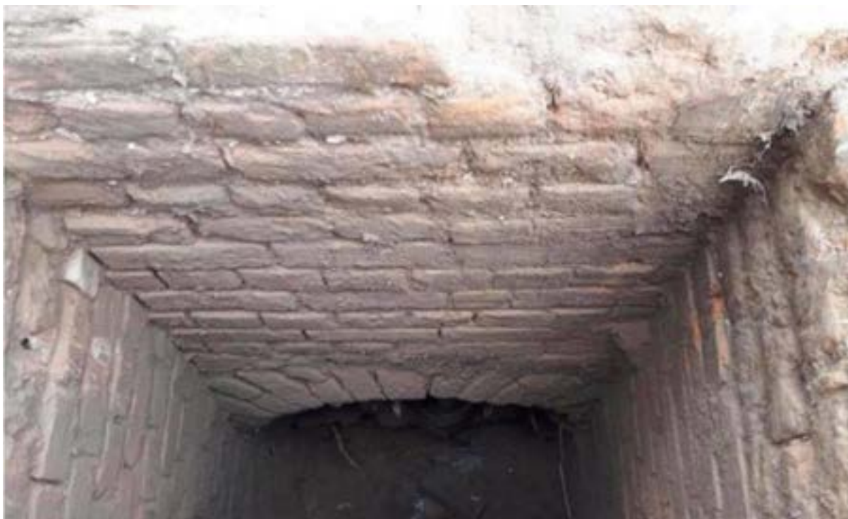
Figure 35 - Brick shaft for the main drain alignment (Source RMS 2018)
