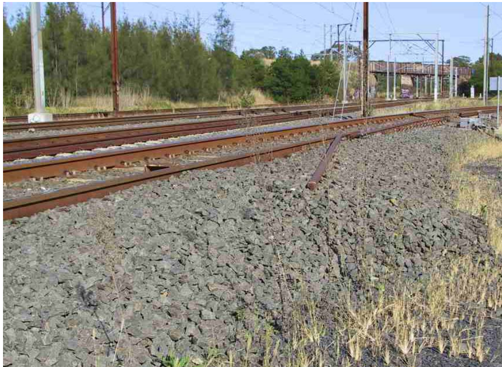
Figure 3 - Example of catchpoint with poor landing zone
