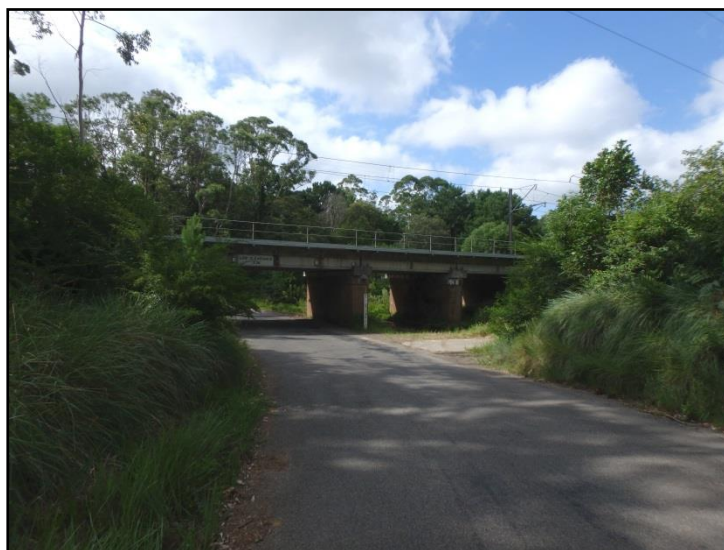
Figure 7: Rail line over Turpentine Road and tributary of Ourimbah Creek. View south-west.
