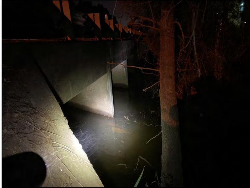
Photo 11. Potential microbat roosting habitat within culverts spanning a non-perennial stream north of the intersection of Mamre Road and Erskine Park Road
