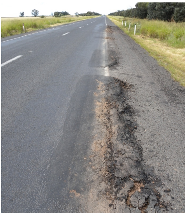
Photo 2-3 Example of heavy patching along the Newell Highway
