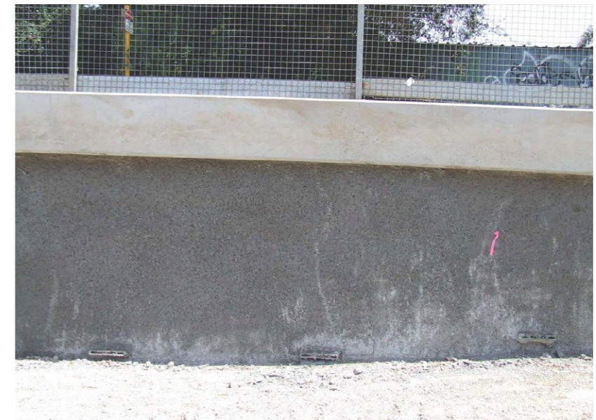
Figure 6-18 Example of gun finish shotcrete and capping beam (for use in areas away from station precincts and for 3:1 vertical face cuts)
