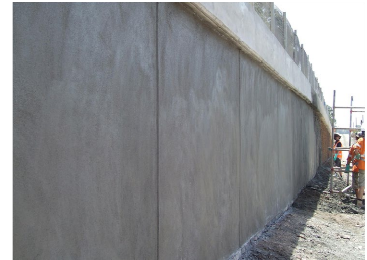
Figure 6-10 Example of wood float and sponge finish with joints at 3m intervals (vertical or 4:1 vertical cut face)
