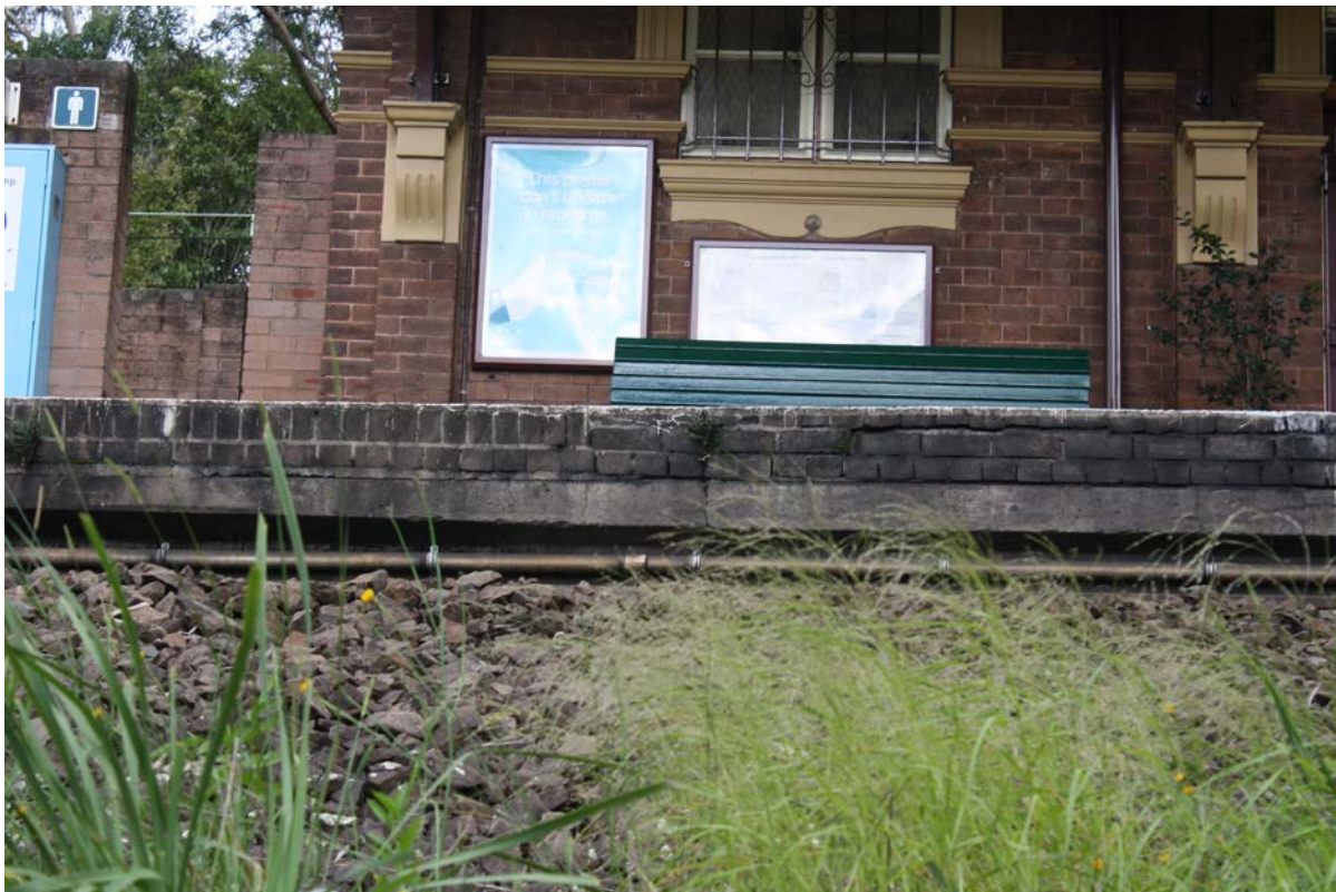
Figure 9 Platform 1 at Woodford Station showing the 1902 concrete coping capped with 1940s brickwork of varying arrangement
