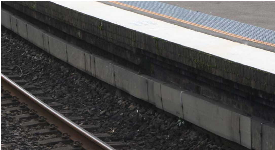
Figure 11 View looking north of the platform 2 at Hazelbrook Station showing the junction between the 1902 and 1940s platform phases
