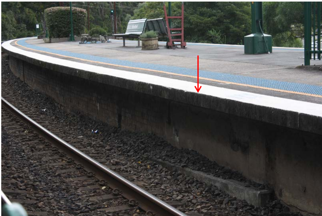
Figure 8 Platform 2 at Woodford Station showing the junction between the 1902 and 1940s platforms, together with the concrete coping. The junction is shown denoted by an arrow
