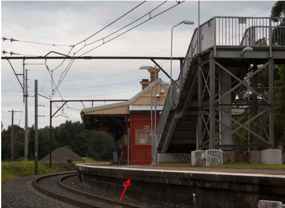
Figure 5 View west of a section of Linden Station platform 1. Note modifications to platform coping denoted by an arrow
