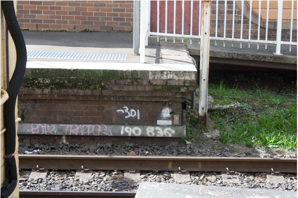
Figure 6 View north of eastern end of platform 2 showing battering of brick platform face. Note lack of concrete coping
