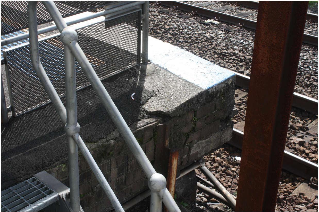
Figure 7 Eastern end of the heritage platform. Note rail used to arrest slumping
