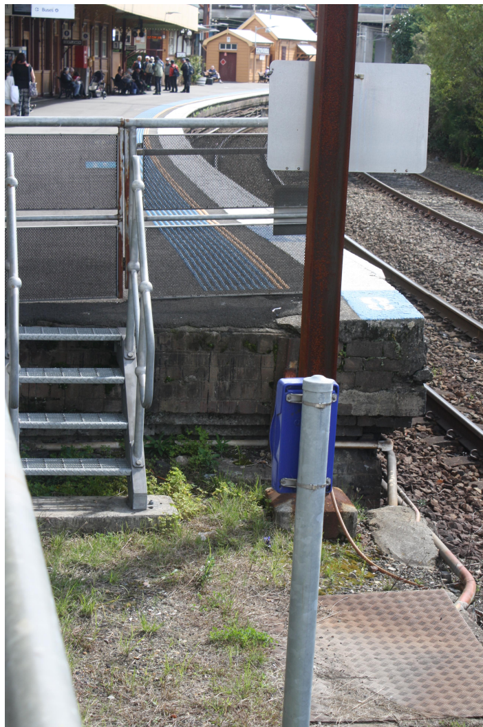
Figure 16 View of gate, stairs and fence proposed for removal at the Sydney end of platform 1
