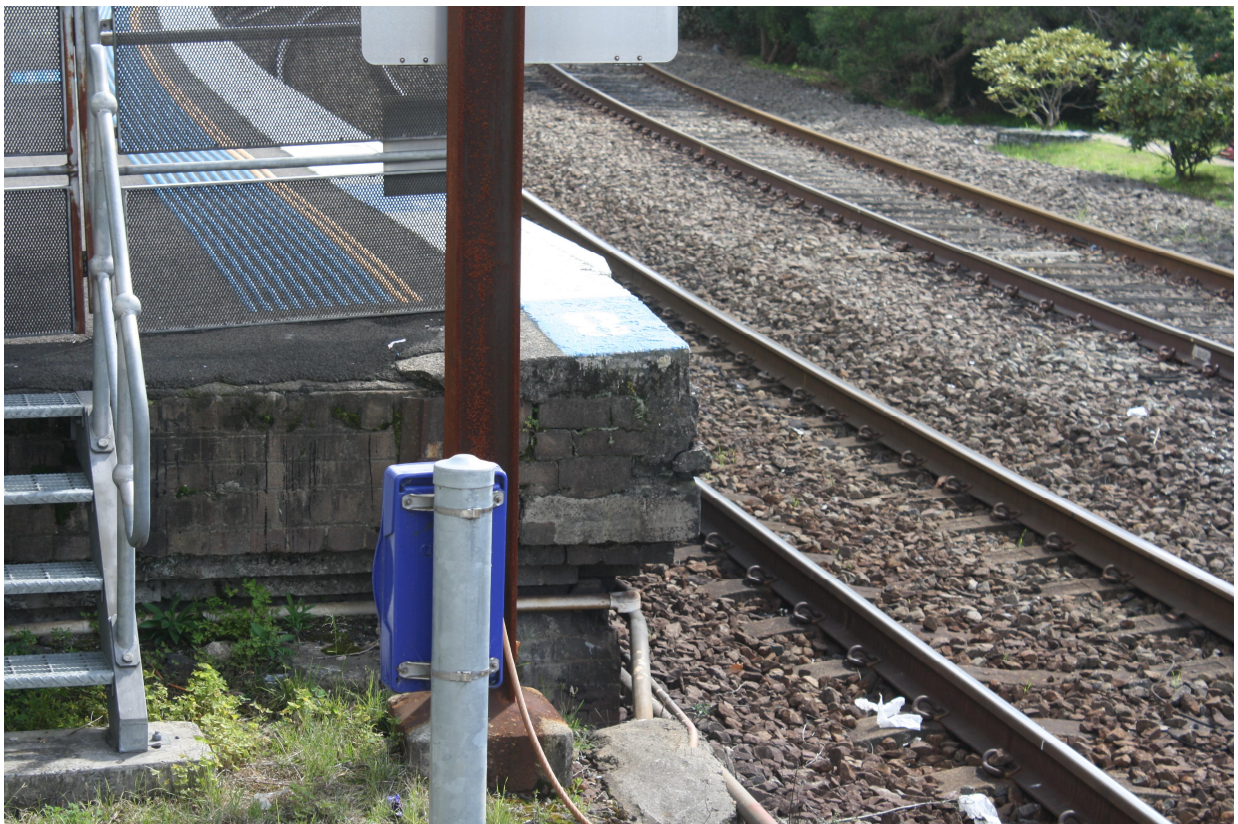
Figure 8 View of tracks near the eastern end of Platform 1. Note concrete coping projecting from edge of platform
