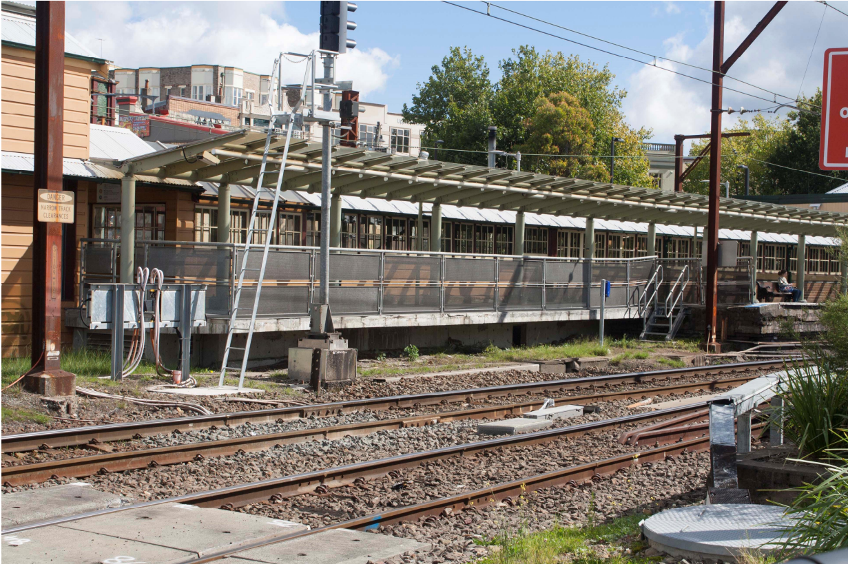
Figure 4 View south west of platform 1, showing junction between the heritage platform and 2009 extension
