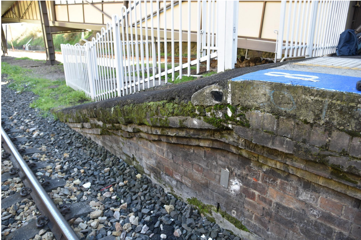
Figure 7: Detail of asphalt covered ramp on southern side of the island platform, showing brick coping extending to rail level
