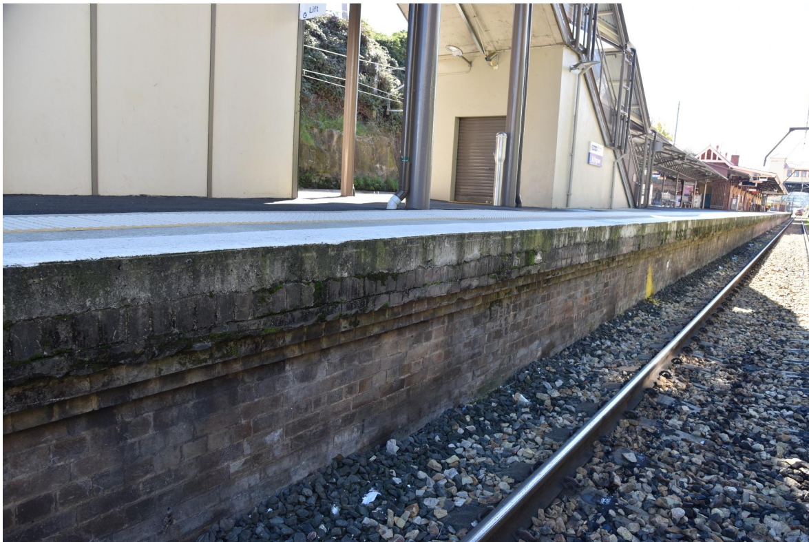
Figure 6: Detail of platform retaining wall, and brick and concrete coping, north-east aspect
