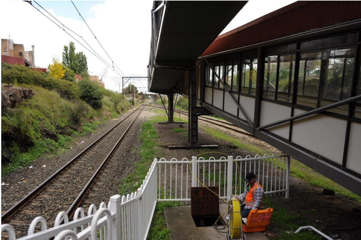
Figure 8: View of western end of rail corridor showing concrete sleepers and service maintenance hatch, west aspect
