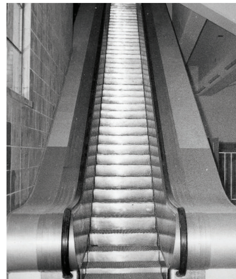
Figure 33: New Otis escalators installed at Circular Quay station. (Source: Australian Railway Historical Society (ARHS))
