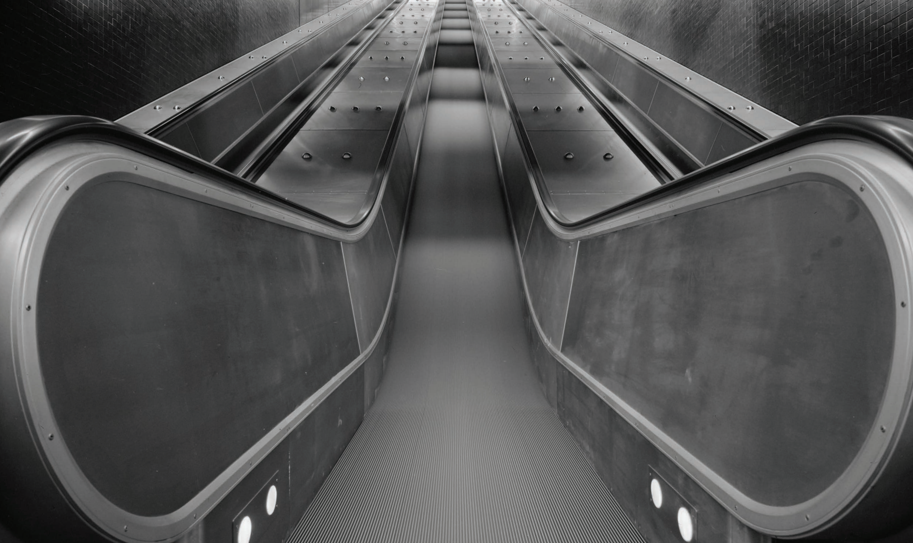
Figure 34: Max Dupain photo of the new 1979 escalators installed at Martin Place Station. (Copyright: Cement Concrete and Aggregates Australia, Supplied: State Library of NSW).
