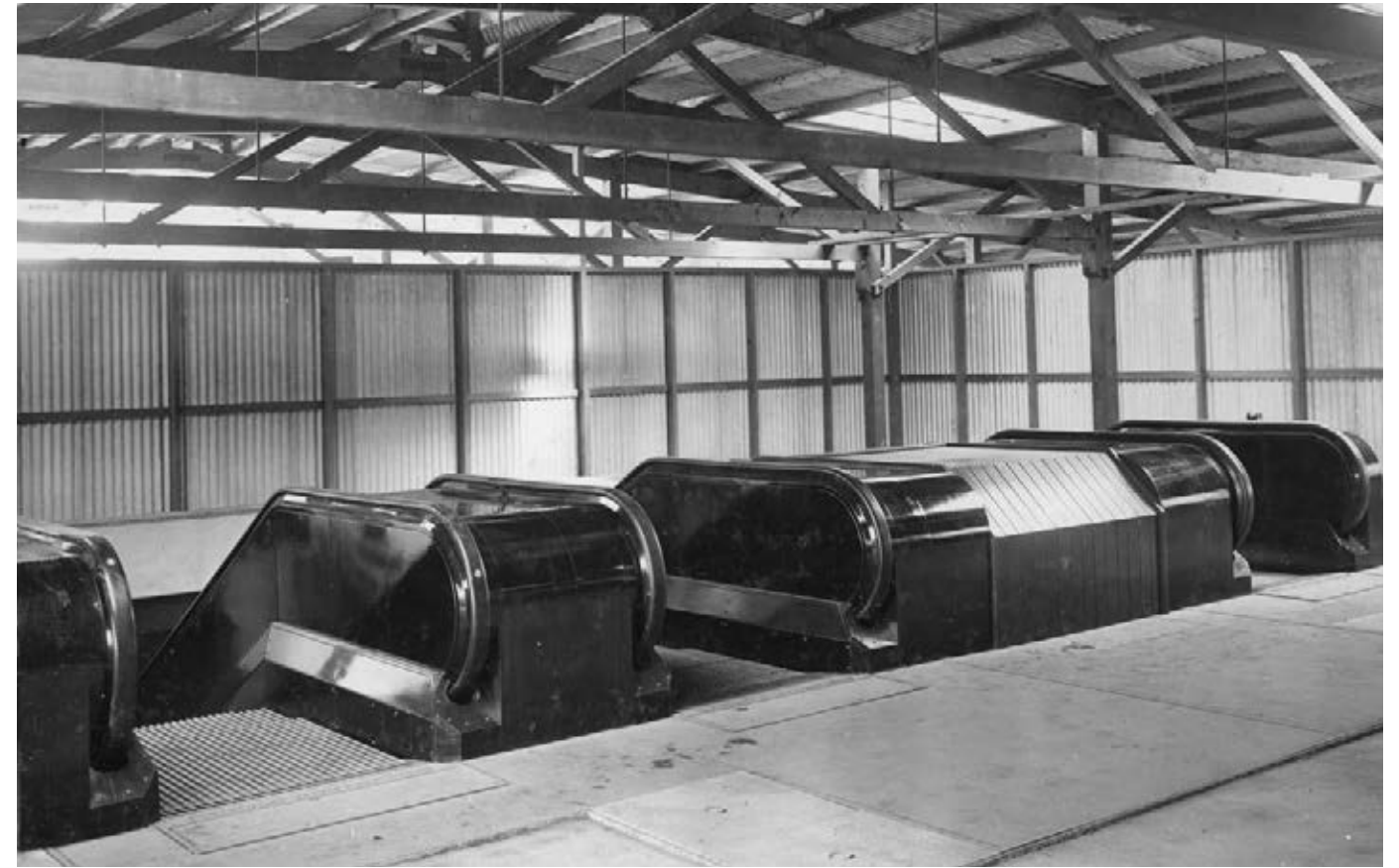
Figure 21: Wynyard Station escalators fully installed and ready for testing in 1931. Note the covered section where future capacity for a fourth escalator was provided. (Source: Sydney Trains)
