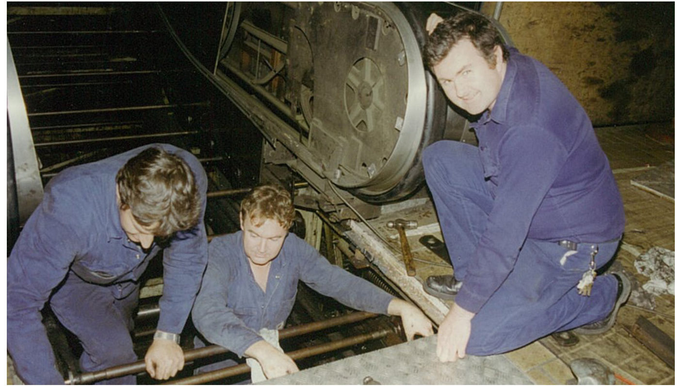
Figure 40: Crew from the Lift and Escalator Section dealing with an urgent escalator problem at Town Hall Station over the Christmas holidays in the 1990s. L-R: Fitters Mal Green, Kevin Taylor and senior foreman Martin King. (Source: Sydney Trains)
