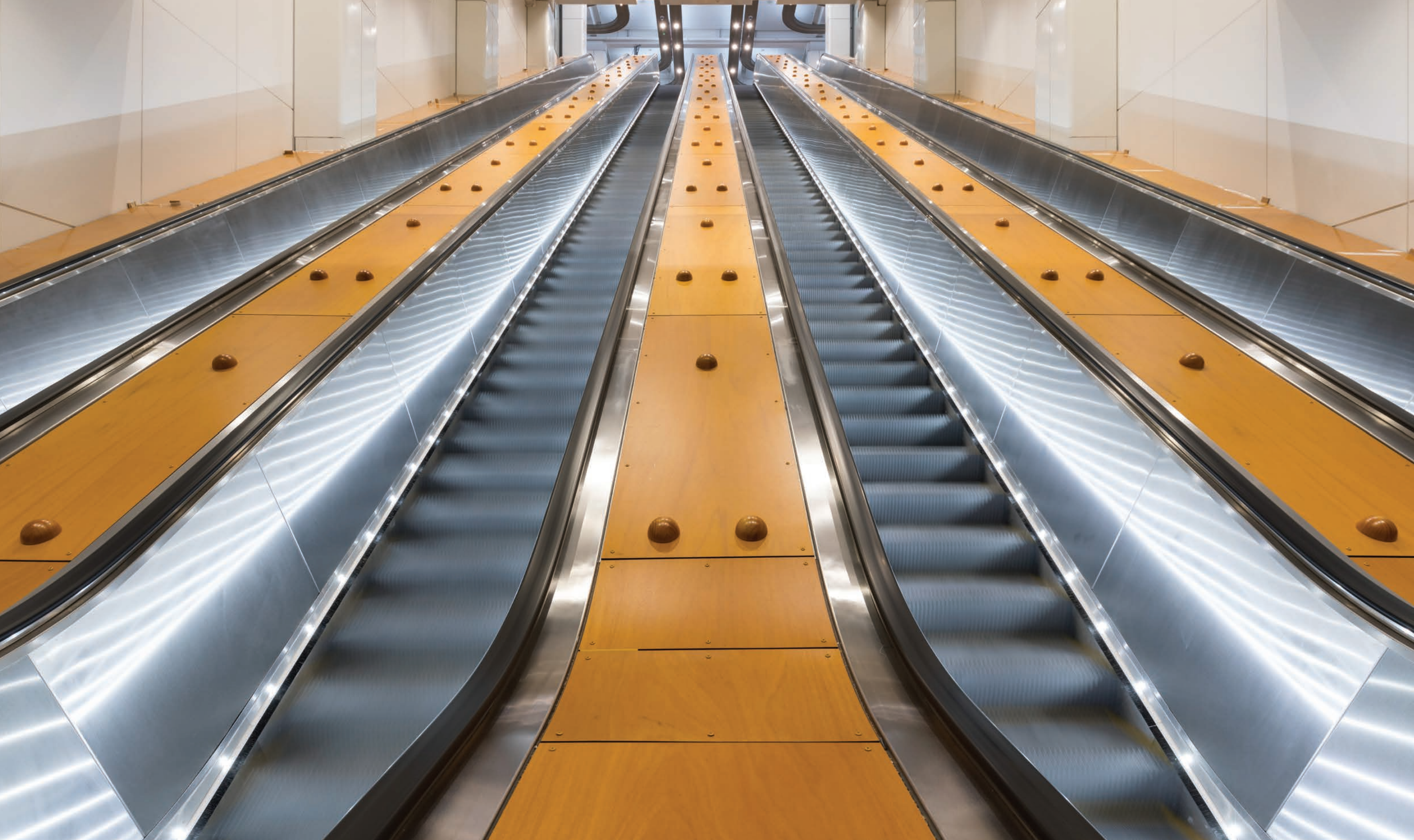
Figure 45: New escalators installed at Wynyard Station in 2017 with metal steps and wood-like decking reminiscent of the historic machines. (Source: Transport for NSW)
