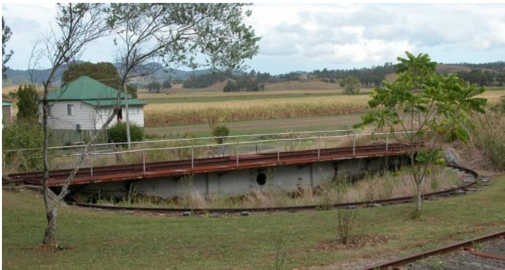
Figure 23. Murwillumbah's 60ft railway turntable circa 2005. Note the lowered side walls and concrete wings below the railway track at either end. (Source: RailNet).
