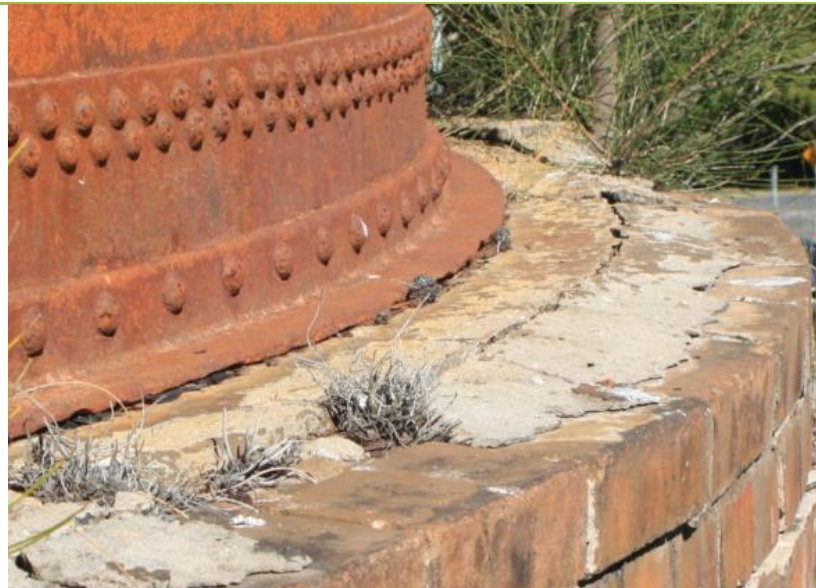
Figure 47. The lower flange attached to the tank and the rendered coping on the brickwork were designed to shed stormwater but both are in poor condition.
