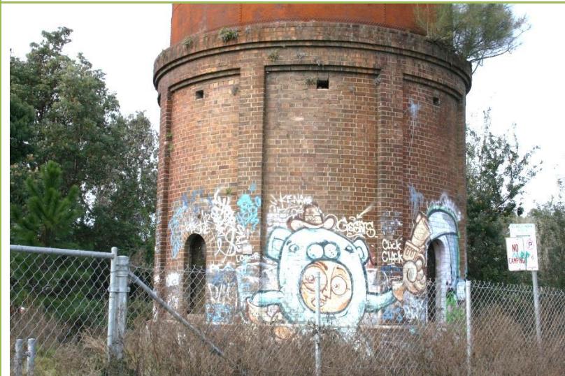
Figure 42. The brick tower is generally in good condition, except where affected by vegetation and metal corrosion around the top.
