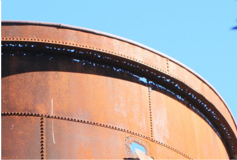
Figure 49. The corrosion of the upper horizontal tank lip appears more advanced than corrosion of the vertical surfaces.
