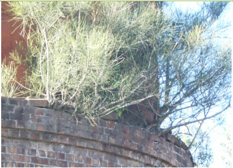
Figure 44. Brickwork around the upper rim is badly affected by vegetation growth.
