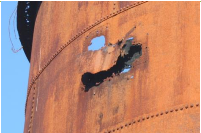
Figure 45. The metal work of the tank already shows evidence of previous corrosion repairs
