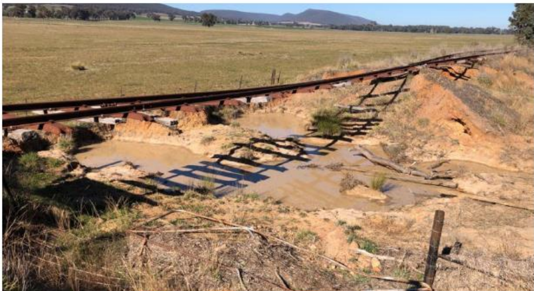
Figure 1 Section of Washaway at approximately 402.300km
