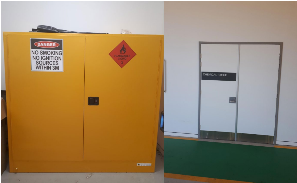
Figure 1 – designated chemical storage room containing bunded chemical and fuel storage containers within maintenance building
