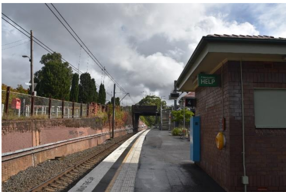
Figure 79: The rear (south-western) elevation of the Shelter Shed on Platform 3/4, view north-west (Source: Artefact 2021)
