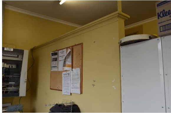
Figure 50: View of the retained portion of an original partition at the north-western end of the office, view north (Source: Artefact 2021)
