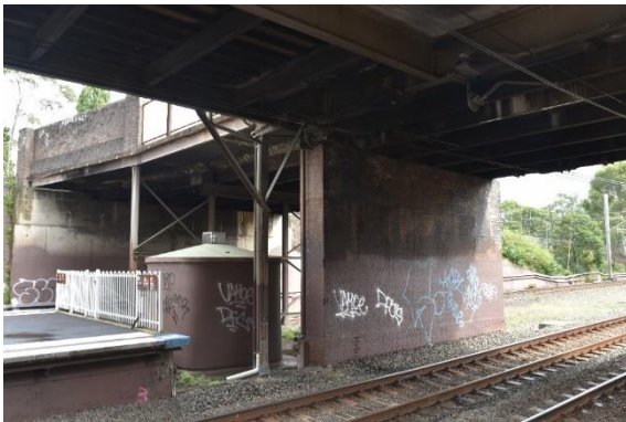
Figure 41: View of the south-western end of the overbridge, showing the brick piers, concrete rendered abutment and steel supports (Source: Artefact 2021)
