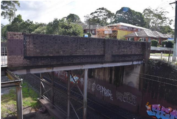
Figure 39: View of the south-eastern side of the overbridge, showing the brick parapet, concrete abutment and steel supports (Source: Artefact 2021)
