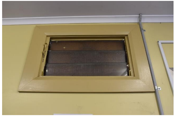
Figure 52: View of the c.1945 clerestory window along the north-eastern elevation, view north-east (Source: Artefact 2021)
