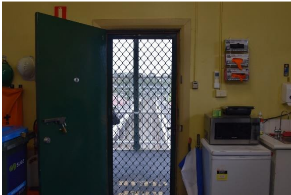
Figure 51: View of the doorway in the south-eastern elevation, view south-east (Source: Artefact 2021)
