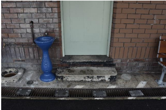
Figure 89: The grated drain along the front elevation of the Conveniences Building on Platform 1/2, view north-east (Source: Artefact 2021)
