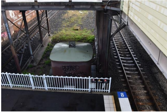
Figure 96: The signal/communications box as viewed from the footbridge on Platform 3/4, view north-west (Source: Artefact 2021)
