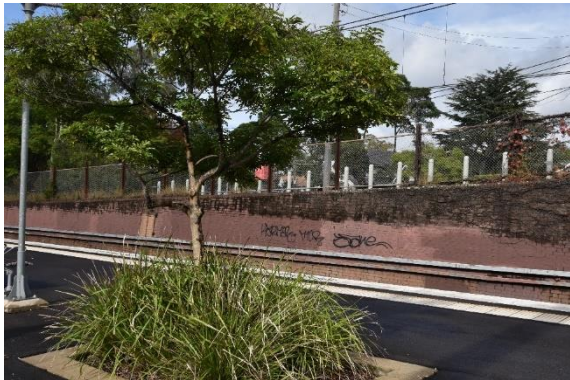
Figure 93: The southern end of the south-western retaining wall from Platform 3/4, view north (Source: Artefact 2021)
