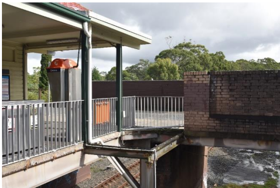
Figure 47: View of the extant steel supports from the former bookstall, view west (Source: Artefact 2021)
