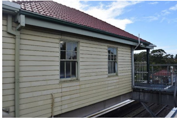
Figure 44: View of the side (south-western) elevation of the overhead booking office from the overbridge, view south (Source: Artefact 2021)
