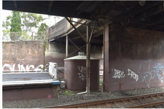
Figure 97: The signal/communications box as viewed from the Platform 1/2, view west (Source: Artefact 2021)
