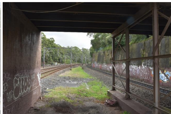
Figure 92: The north-eastern retaining wall to the north of the station from the end of Platform 1/2, view north-west (Source: Artefact 2021)
