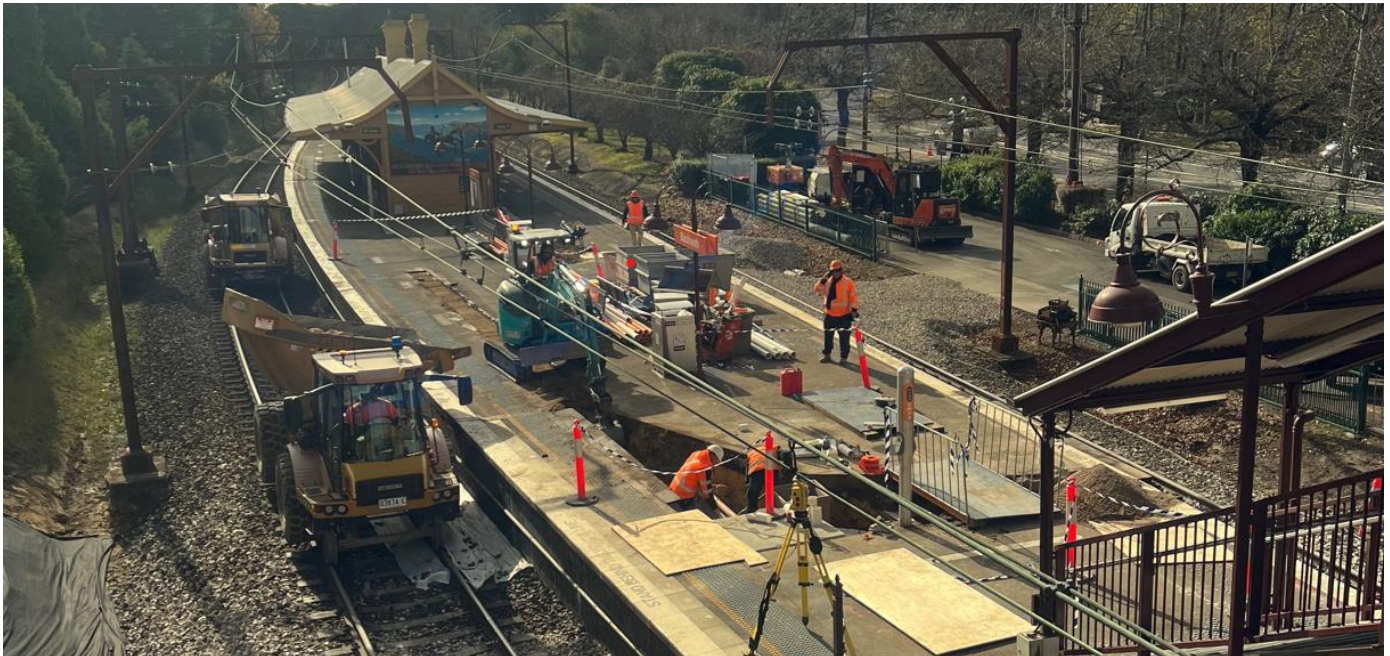
Above: Works progressed in recent months to install services for the new lifts and station building at Blackheath Station.
