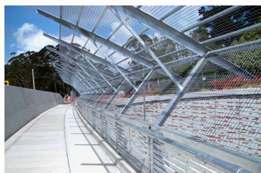
New fences and safety screens introduce new and aggressively different design treatments that have little to do with their context
