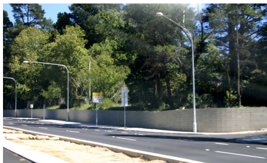
New consistent height retaining walls in front of the Blue Mountains Grammar School
