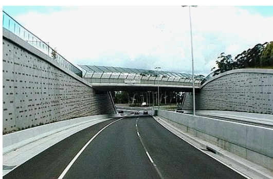
There is an uncomfortable union between the complex retaining wall brick inlay patterns, the irregular form of the cutting walls and the new elegantly curved bridge soffit.
