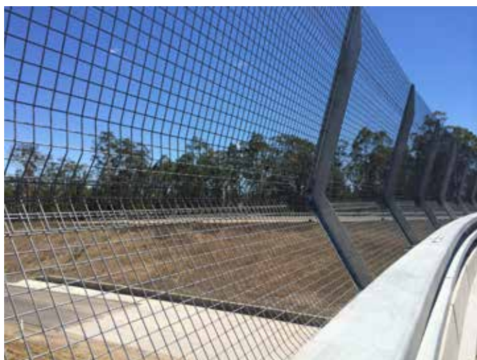
▲ HUNTER EXPRESSWAY CRANKED STEEL BEAM SAFETY SCREEN
