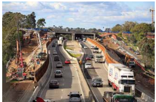
Work on the new M2 on and off ramps at Windsor Road, Baulkham Hills, June 2011.
