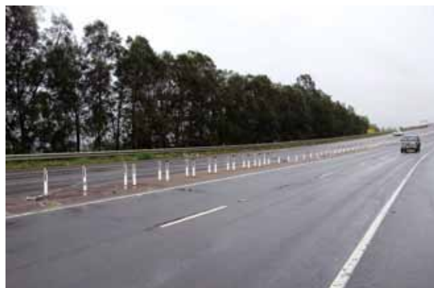
Wire rope safety barriers on the New England Highway at Maitland, November 2010.
