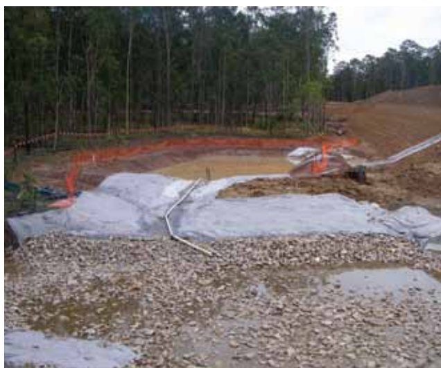
Dewatering a sediment basin via siphoning on the Pacific Highway Upgrade at Glenugie.
