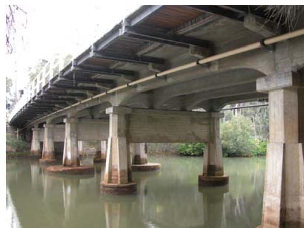
Fullers Bridge ( Bridge No 105) Note curved beam soffit, continuous over piers, providing deeper beams where the bending moments are greatest
