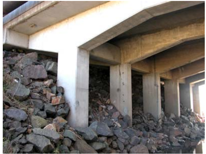
Stapletons Bridge Albion Park (RTA Bridge No 881) showing original frames, centre, and widening frames
