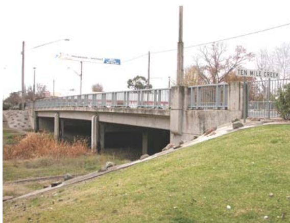
Ten Mile Creek, Holbrook (RTA No 5444) In town centre with model rail track beneath.
