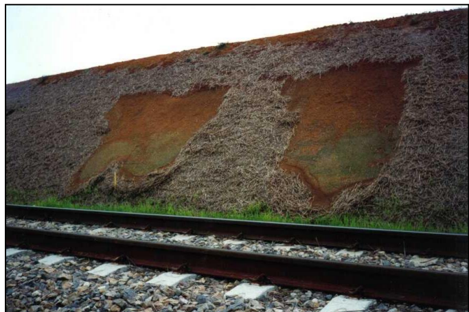
Figure 7. A steep smooth cutting is difficult to stabilise.
