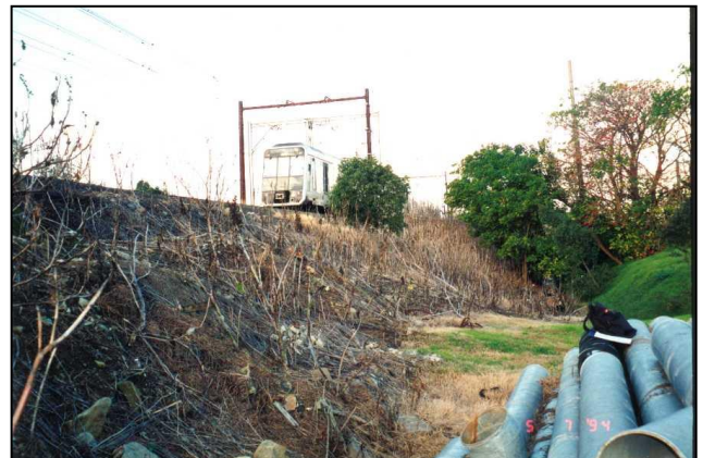
Figure 20. This rail embankment at Sydenham is regularly sprayed to control the continual growth of castor oil, a Noxious Weed. Such practice is unsustainable and very expensive. A long-term solution would be to progressively revegetate this area with local native shrubs.
