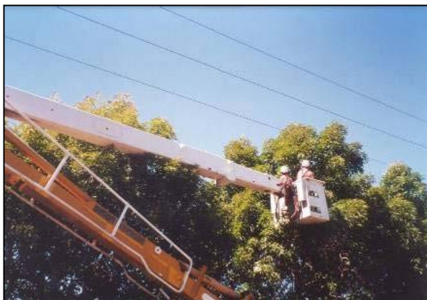
Figure 17. Clearing under powerlines is both expensive and time consuming. The ultimate height of the tree must be considered before planting under or near any electrical powerlines or overhead wiring.
