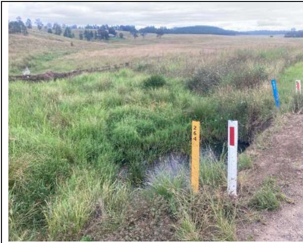
Plate 1: Box culvert 264 at eastern end of site will require headwalls to be extended.
