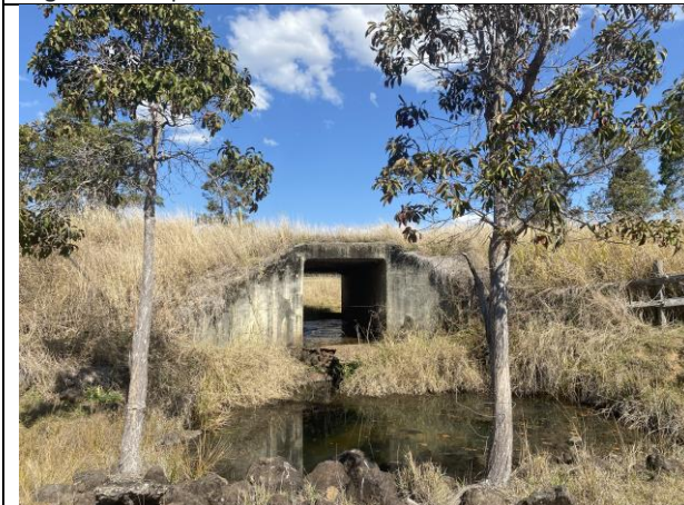
Plate 5: Culvert extension required at ch 48775. The two small Swamp Box will require removal; dewatering of the small pond will also be required.
