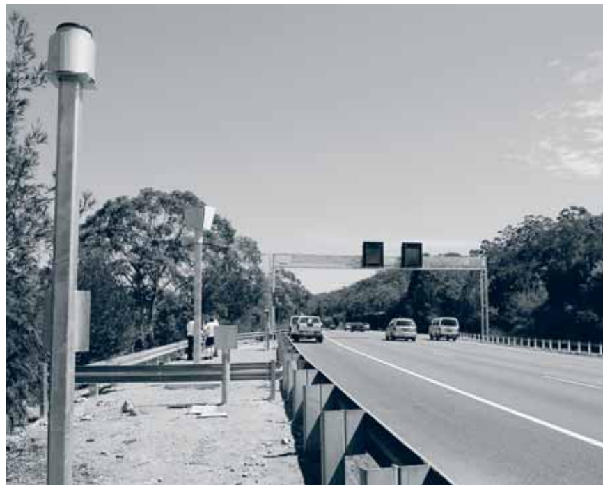
Signage and technology designed to automatically reduce speed limits during wet weather was introduced on the F3 freeway at Mount White.
