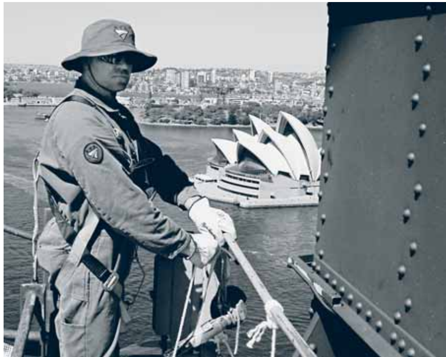
Chris Mihellis installing containment for lead paint removal on the lower chord of the Sydney Harbour Bridge.
