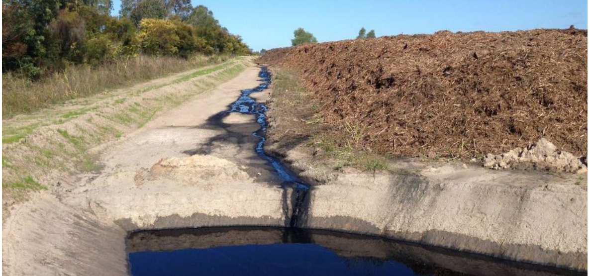
Figure 4.5: Management of mulch tannins from the Woolgoolga to Ballina Upgrade Pacific Highway (Photo: Anthony Arena, TfNSW)
