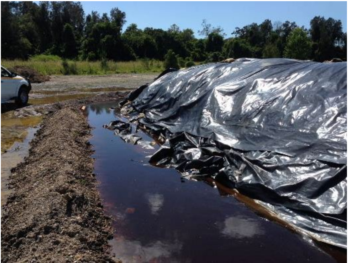
Figure 7.8: Soil solarisation to control soilborne pathogens using high temperatures on the Woolgoolga to Ballina Upgrade of the Pacific Highway) (Photo: Anthony Arena, TfNSW).
