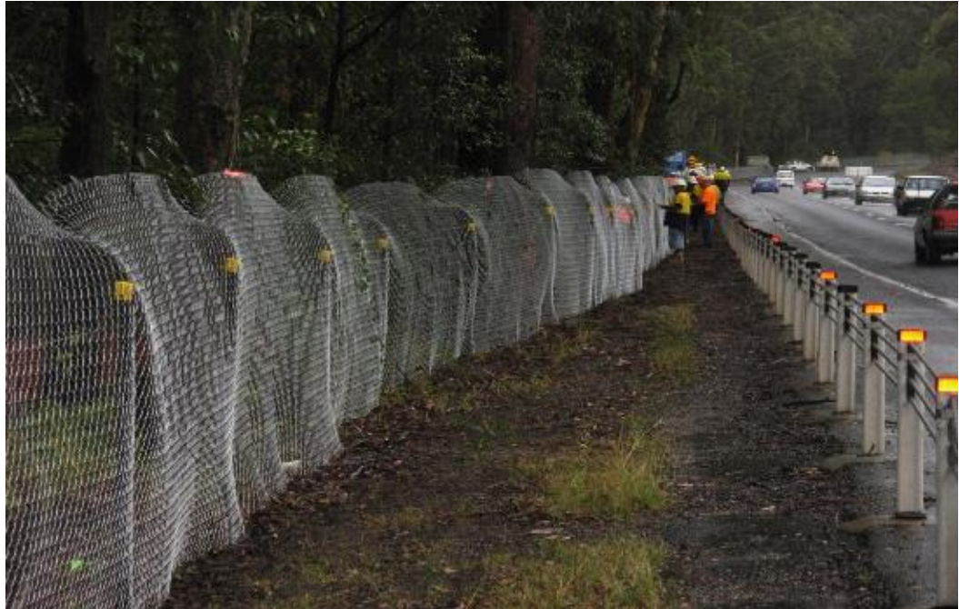
Figure 2.4: Example of temporary construction fauna exclusion fencing targeting koala on the Bonville Pacific Highway Upgrade Project (Photo: Scott Lawrence, TfNSW).
