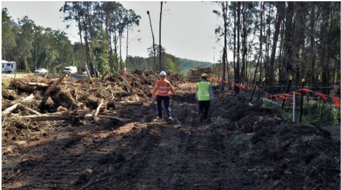
Figure (ii): Clearing native vegetation has the potential to cause unintended impact on biodiversity. When clearing native vegetation, refer Guide 4: Clearing of vegetation and removal of bushrock (Photo: Anthony Arena, TfNSW).
