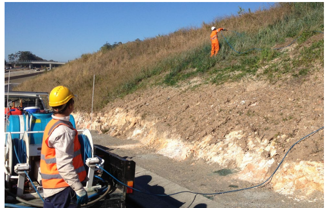
Figure 6.5: Herbicide application by foliar spraying on the Sapphire to Woolgoolga Pacific Highway Upgrade Project (Photo: Envite).
