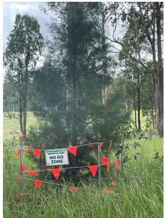
Figure 2.2: Exclusion fencing around a retained threatened Bailey's Cypress Pines ( Callitris baileyi ) on the Bruxner Highway (Photo: Ben Christiansen, TfNSW).
