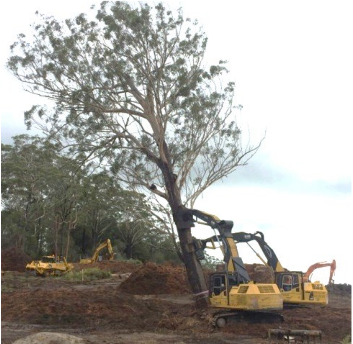
Figure 4.8: Habitat tree being carefully felled and lowered by excavators during the second stage of clearing for the Nambucca Heads to Urunga Pacific Highway Upgrade (Photo: Sandpiper Ecological Surveys).
