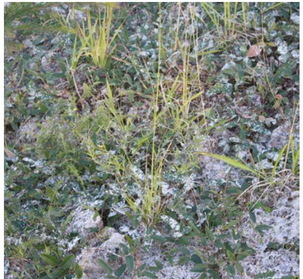
Figure 3.5: Diverse vegetation establishment resulting from hydroseeding overlaid with hydromulch on the Kempsey Bypass. (Photo: TfNSW).
