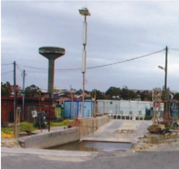
Figure 7.9: Wheel wash bay used at Tempe Reserve during construction of the Airport Link, Sydney Region. Most trucks drove through the wheel wash, but some vehicles needed to be scrubbed so that materials were not transported from site. The water depth was approximately 400mm, with a cattle grate underwater for solids to settle under (Photo: Leigh Trevitt, TfNSW).
