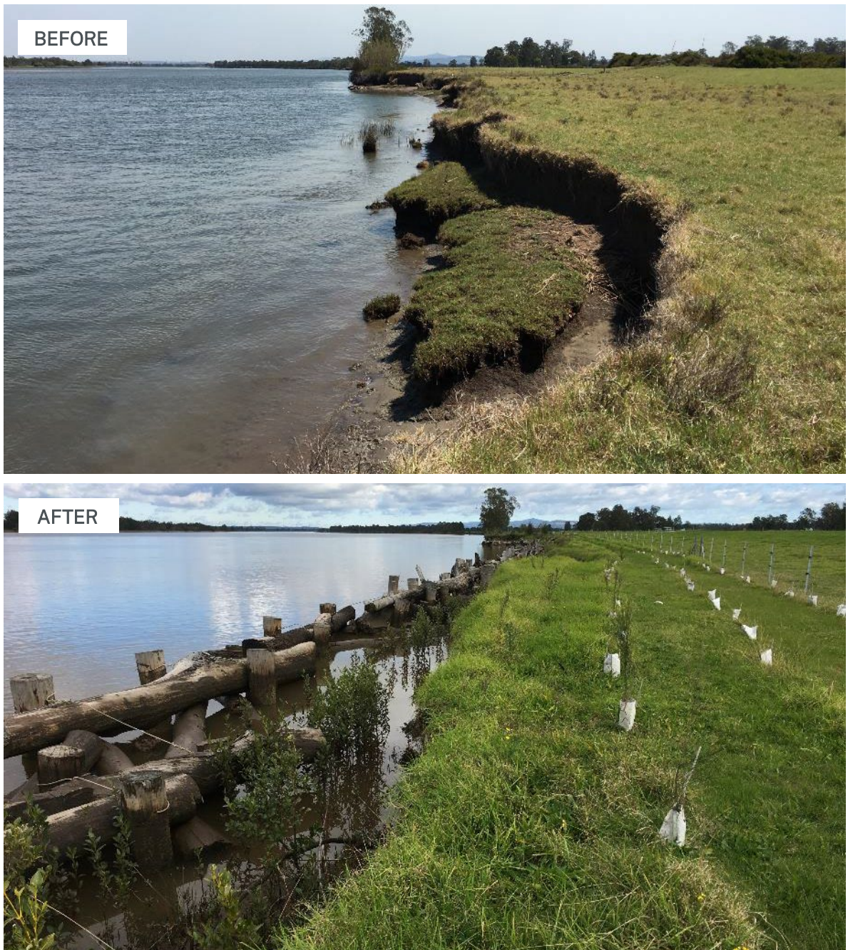
Figure 10.7: Before (above) and after (below) bank erosion management on the Hunter River at Millers Forest 2018-2020. Log walls were constructed from large woody debris salvaged during vegetation clearing (Photos: LLS).
