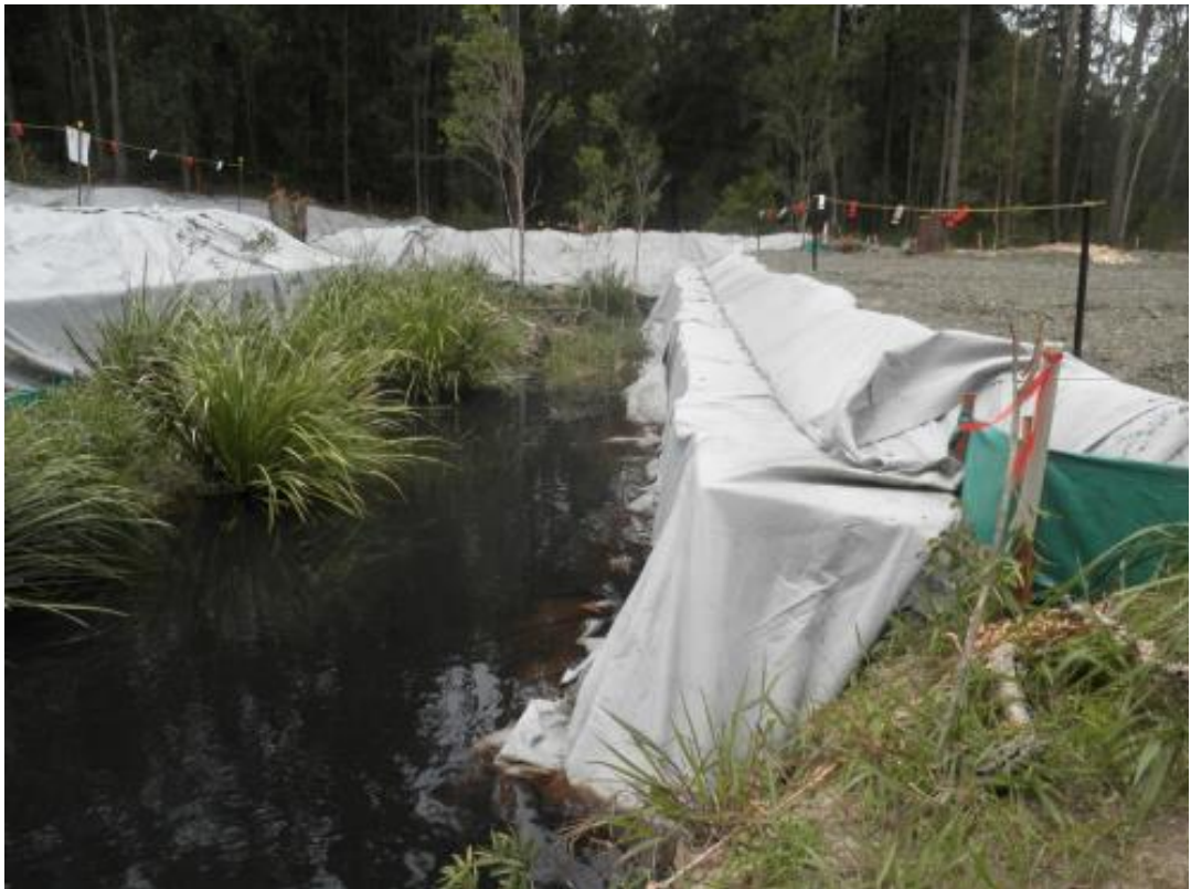
Figure 10.2: Working in riparian zones requires measures to protect the waterway, including geofabric to control erosion/sedimentation and exclusion fencing (Photo: TfNSW).
