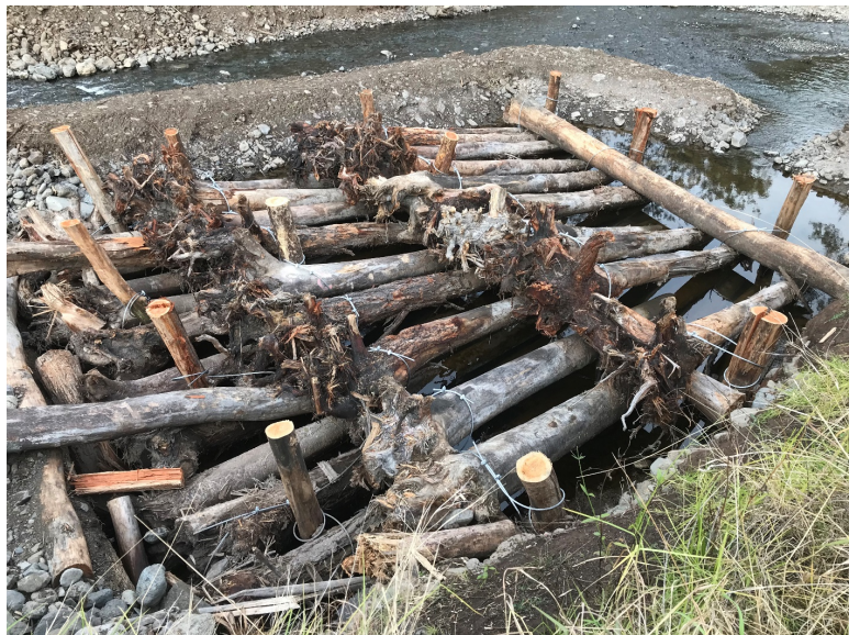
Figure 10.4: An Engineered Log Jam (ELJ) constructed using 'pin logs' and 'rootball logs' salvaged during clearing works creates aquatic habitat and protects from bank erosion achieving good river health outcomes (Photo: LLS).
