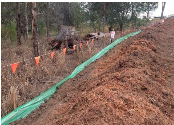
Figure 2.1: Example of mulch bund and construction flagging delineating the construction zone from the environmental protection area (Photo: Anthony Arena, TfNSW).
