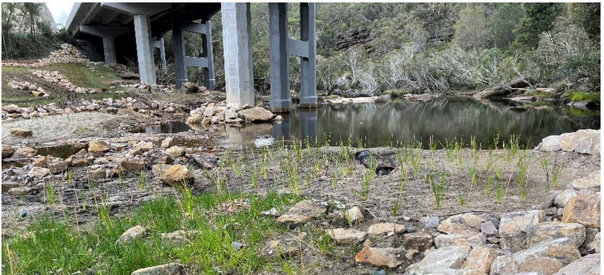
Figure 10.6: Planting wetland species and placement of rock within the Woronora River to reestablish aquatic habitats following completion of the Heathcote Road Bridge upgrade (Photo: Julie Ravallion, TfNSW).
