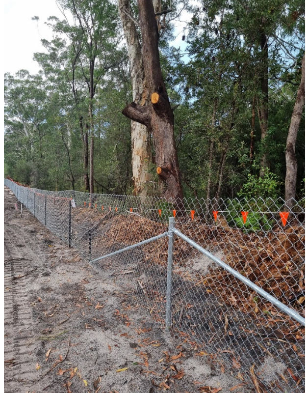
Figure 2.3: Example of temporary construction fauna exclusion fencing on the Nelson Bay Road Upgrade (Photo: Elle Hutchinson, TfNSW).
