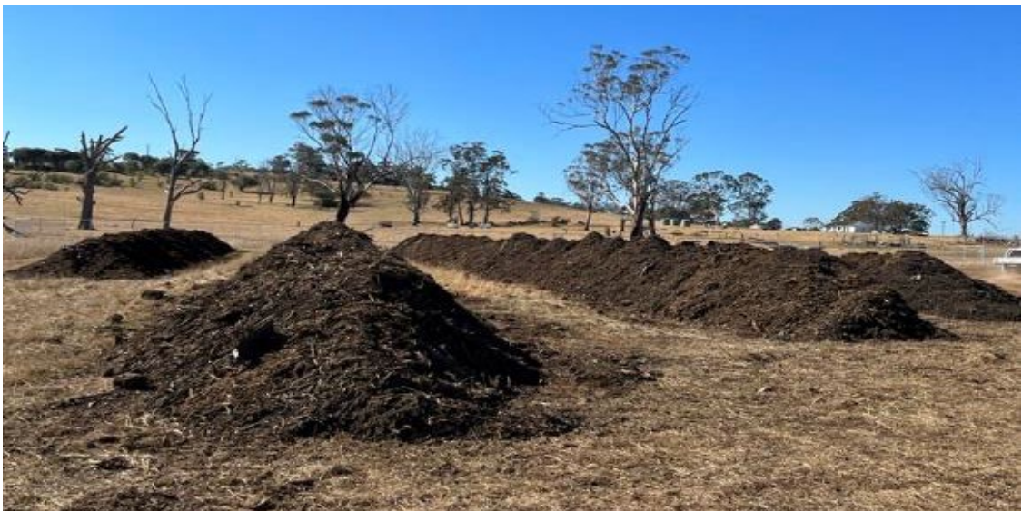
Figure 6.6: Windrows of weed-contaminated mulch are composted onsite for the Spring Farm Parkway Stage 1 Project. Composting creates high temperatures that can destroy organic toxins, weeds seeds and plant propagules and disease organisms (Photo: Amanda Berger, TfNSW).
