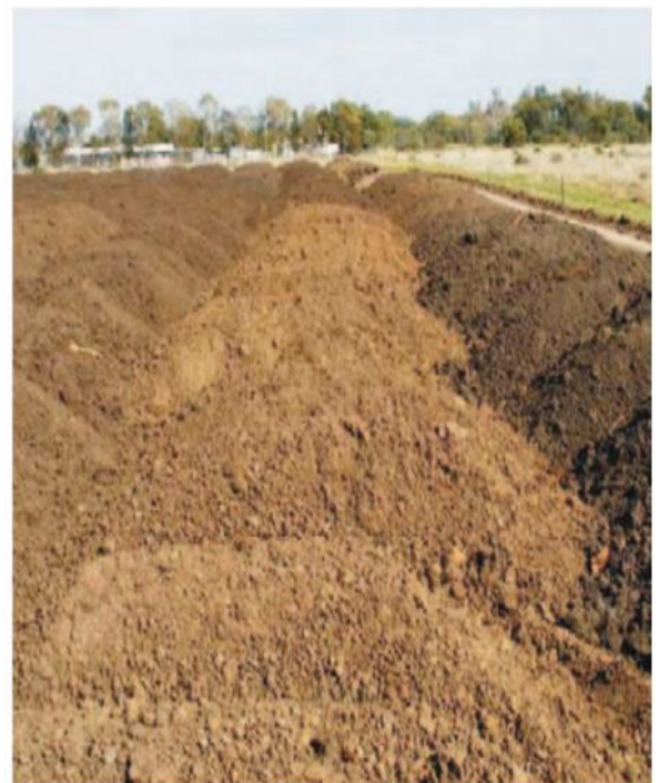
Figure 3.3: Topsoil being stockpiled at Moree for re-use later in revegetation and landscaping works (Photo: Lester Piggott, TfNSW).
