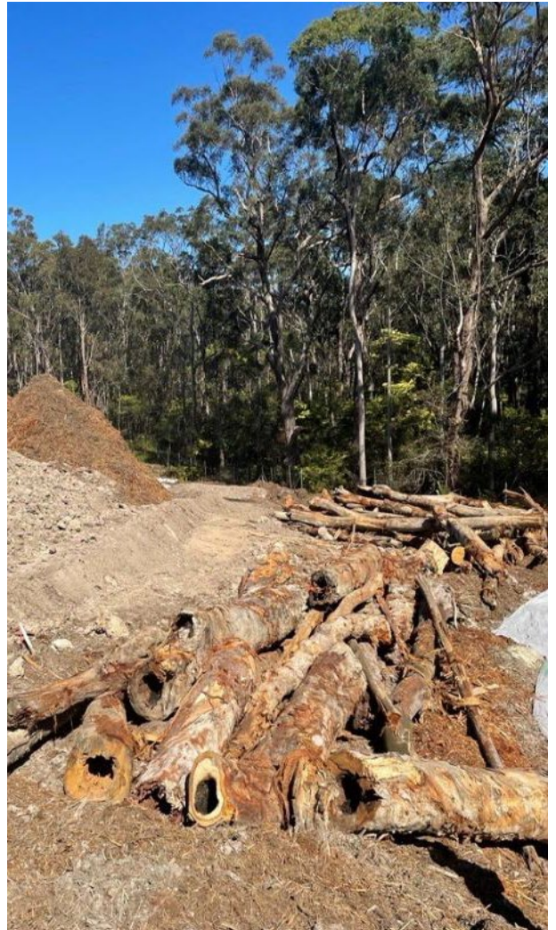
Figure 5.3: Hollow logs retained during clearing and stockpiled for relocation as fauna habitat on the Rankin Park to Jesmond Inner-city Bypass Project (Photo: Rebecca Vaughan, TfNSW).
